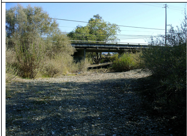
Photo 10: View looking east along the Ackerman Creek bed.
