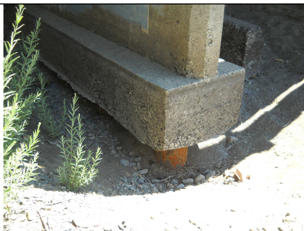
Photo 11: View of scour at one of the bridge piers.
