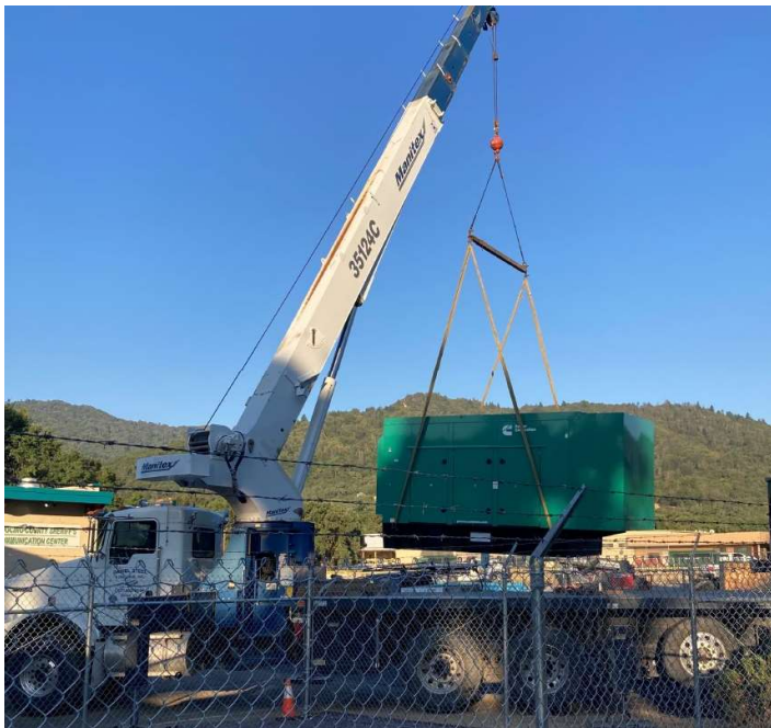
CDBG funded generator being delivered for the 911 Bunker
