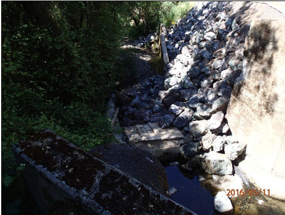
Photo 3. Collapsed Retaining Wall, Viewing from Overbank Area (May 11, 2016)
