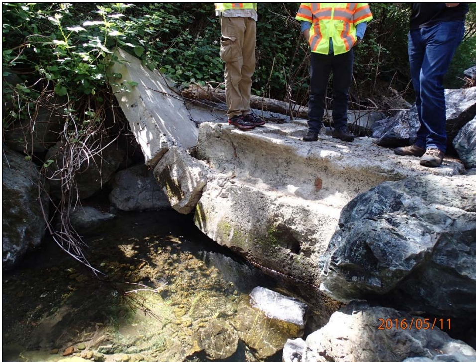
Photo 4. Collapsed Retaining Wall, View from Bottom of Channel (May 11, 2016)
