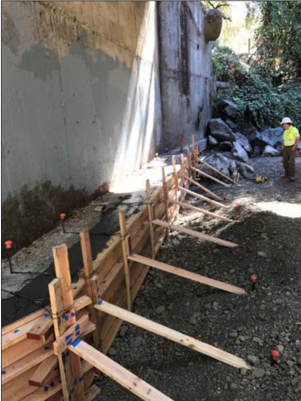
Photo 7. Scour Repair at Abutment 2 (Sept 27, 2017)
