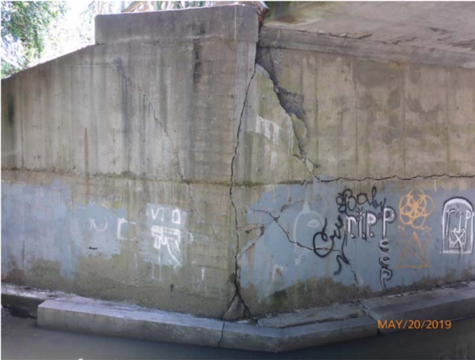
Photo 8. Abutment 2 Failure, Downstream Face (May 20, 2019)
