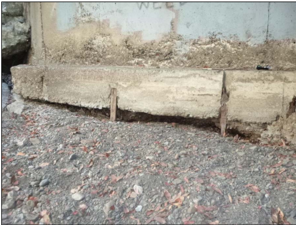
Photo 6. Undermined Footing of Abutment 2 (Eastern Abutment) (Sept 27, 2017)
