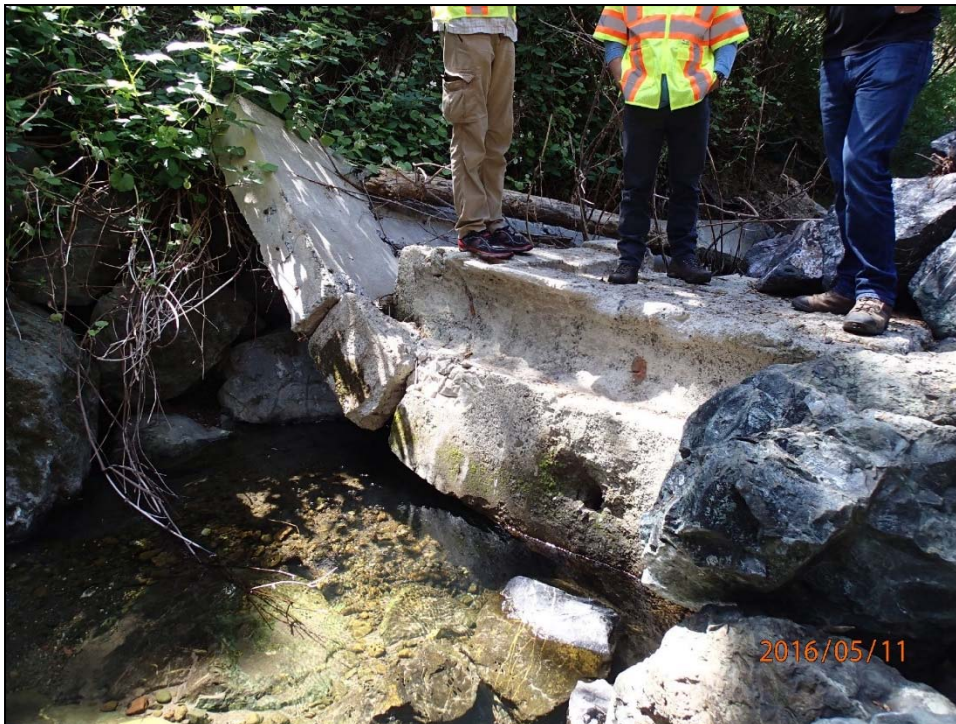
Photo 4. Collapsed Retaining Wall, View from Bottom of Channel (May 11, 2016)
