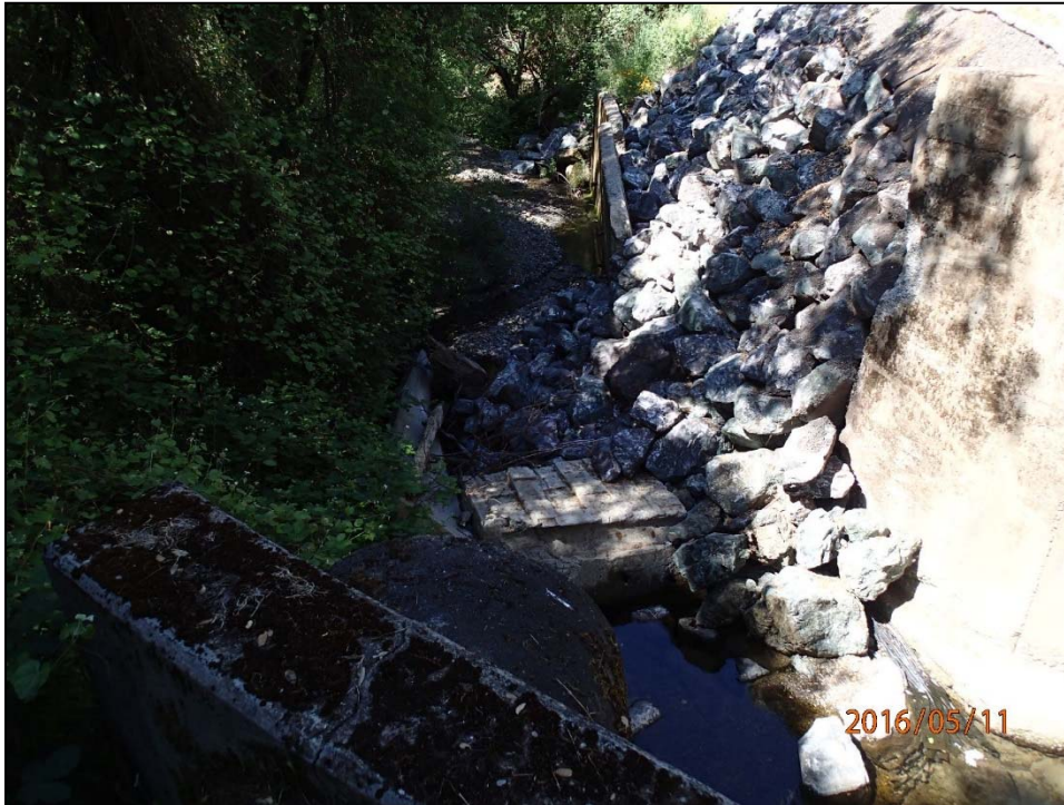
Photo 3. Collapsed Retaining Wall, View from Overbank Area (May 11, 2016)
