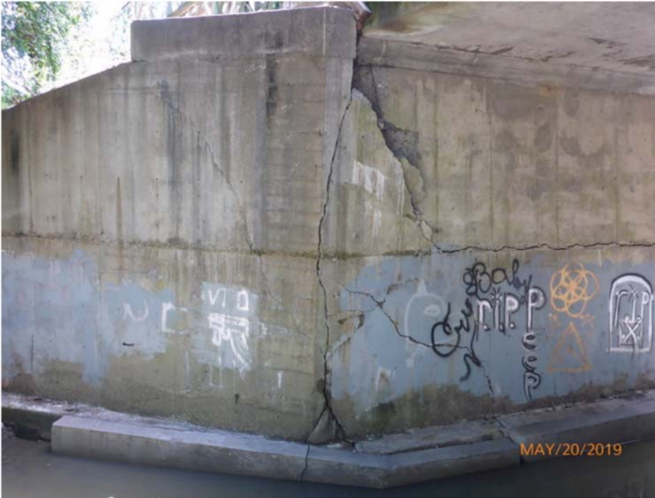
Photo 8. Abutment 2 Failure, Downstream Face (May 20, 2019)
