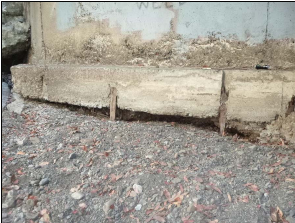
Photo 6. Abutment 2 Undermined Footing (September 27, 2017)
