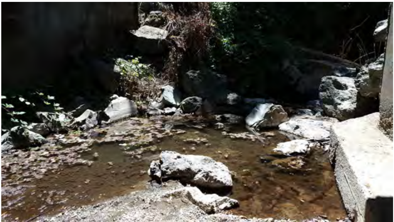
Looking southeast immediately upstream of the bridge at ponded water with algae bloom. The start of the failed retaining wall and RSP that are acting as a fish passage barrier can be seen on the right.
